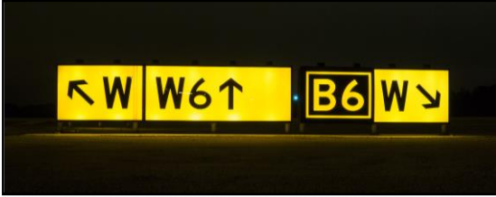
Taxiway Location and Direction Sign (Complex Intersection)
