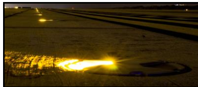
In-Pavement Runway Guard Light
