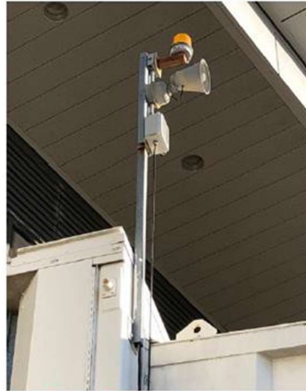
Horn & Beacon (exterior)
