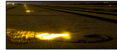
In-Pavement Runway Guard Light
