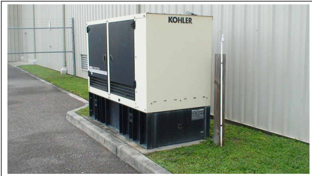
SITE PHOTOGRAPH: DIESEL GENERATOR AST
