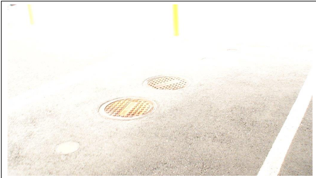
SITE PHOTOGRAPH: OIL/WATER SEPARATOR
