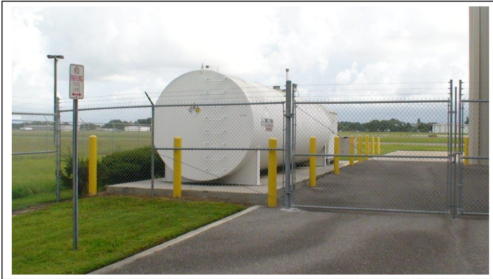
SITE PHOTOGRAPH: JET FUEL AST
