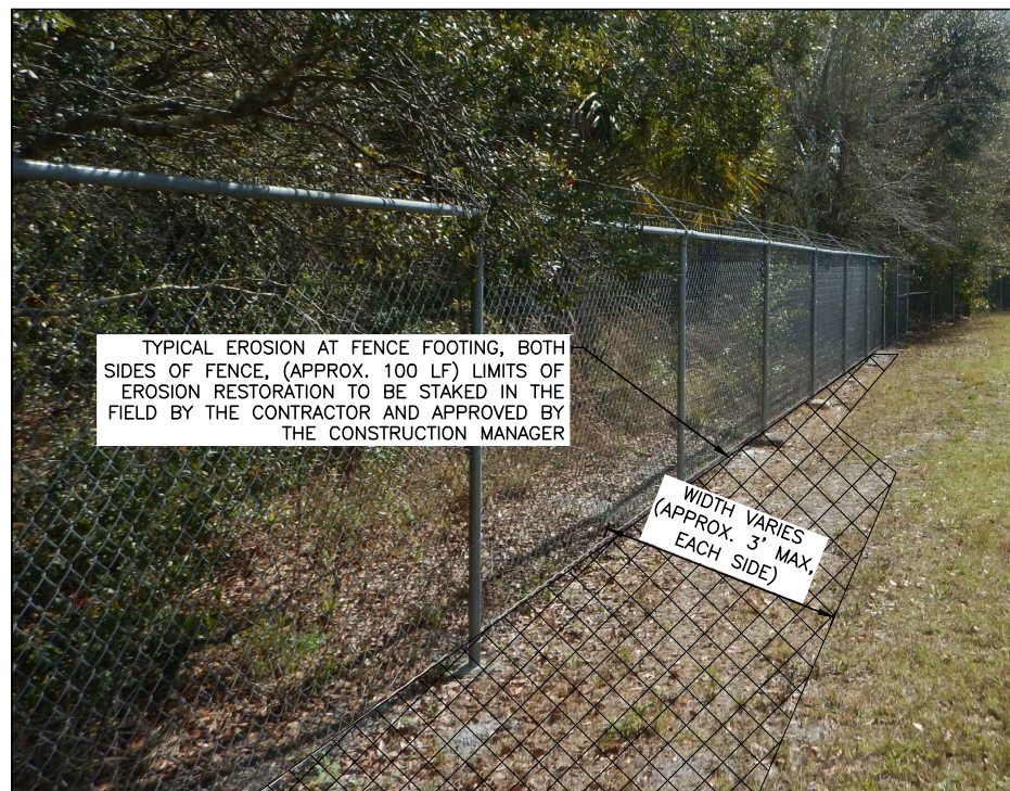
3 FENCE FOOTING EROSION PHOTO C103
