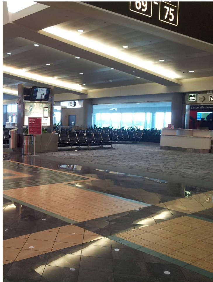
Central zone looking southwest: This is a typical ceiling condition where the ceilings align with the column bays forming room size zones for each gate lounge.
