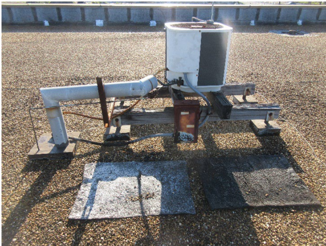
Photo 3 – Typical RTU configuration.
