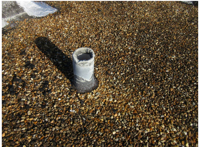
Photo 4 – Typical plumbing vent.
