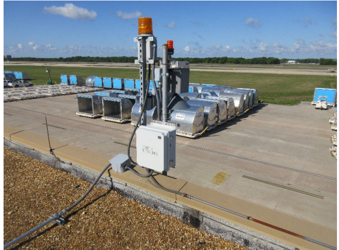
Photo 10 – View of antenna reset at roof area D.
