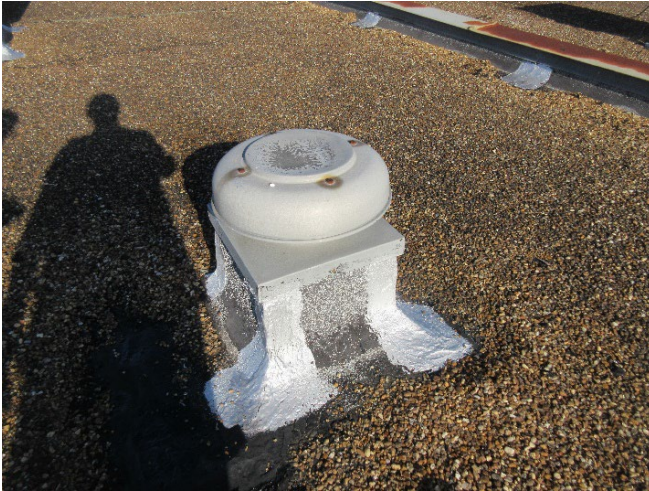
Photo 5 – Typical exhaust fan.
