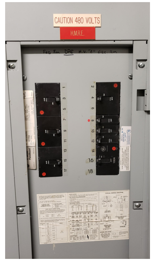
2 1. PANEL HMRE 2. RELABEL 50A/3 BREAKER FOR RTU-7 AS SPARE
