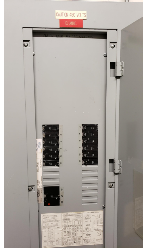
1 1. PANEL EHMRE 2. ADD (1) 15A/3 FOR NEW INTERIOR FOR FCU-P3 AND (1) 15A/3 BREAKER FOR EXTERIOR CU-P3 TO NEW PANEL.
