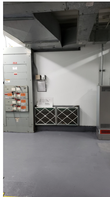
5. 1. INTERIOR WALL AT NEW FCU LOCATION AND ROOM FOR NEW DISCONNECT AT WALL FOR FCU.
