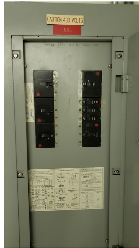
1. PANEL HMRB 2. RELABEL 50A/3 BREAKER FOR RTU-5 AS SPARE
