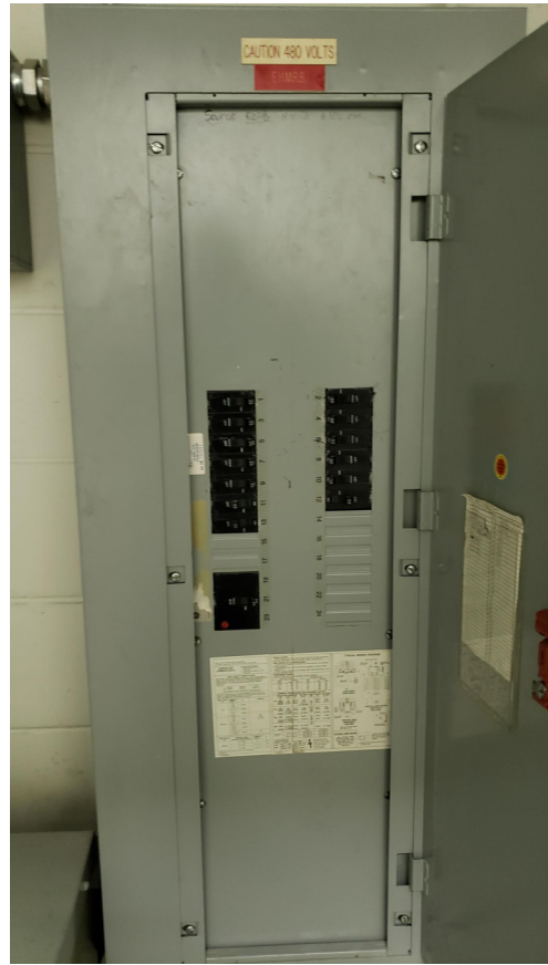
1. PANEL EHMRB 2 ADD (1) 15A/3 FOR NEW INTERIOR FOR FCU-P1 AND (1) 15A/3 BREAKER FOR EXTERIOR CU-P1 TO NEW PANEL.
