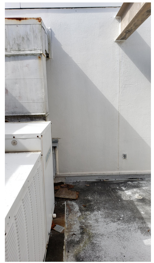
5 1. EXTERIOR WALL AT NEW CU LOCATION AND WALL AREA FOR NEW DISCONNECT AT WALL FOR CU.
