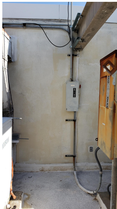
1. EXTERIOR WALL AT NEW CU LOCATION AND WALL AREA FOR NEW DISCONNECT AT WALL FOR CU.
