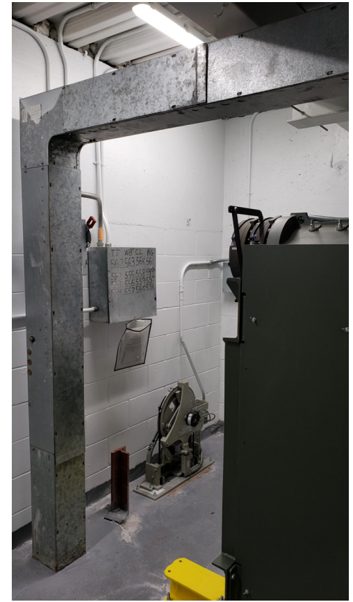
4 1. INTERIOR WALL AT NEW FCU LOCATION AND ROOM FOR NEW DISCONNECT AT WALL FOR FCU.
