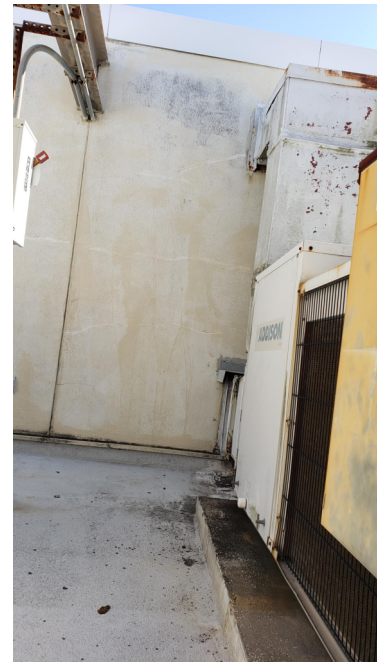
6. 1. EXTERIOR WALL AT NEW CU LOCATION AND WALL AREA FOR NEW DISCONNECT AT WALL FOR CU.
