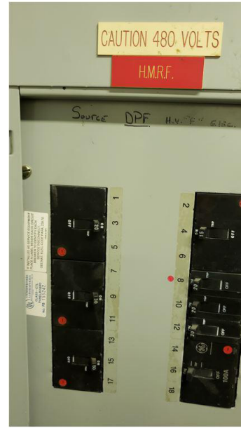
3. 1. PANEL HMRF (50A/3 RTU-7 WILL REPLACE TO SPARE).
