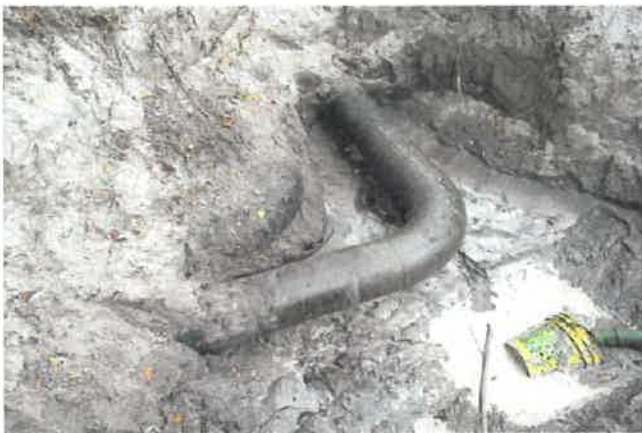
12-inch Piping View
